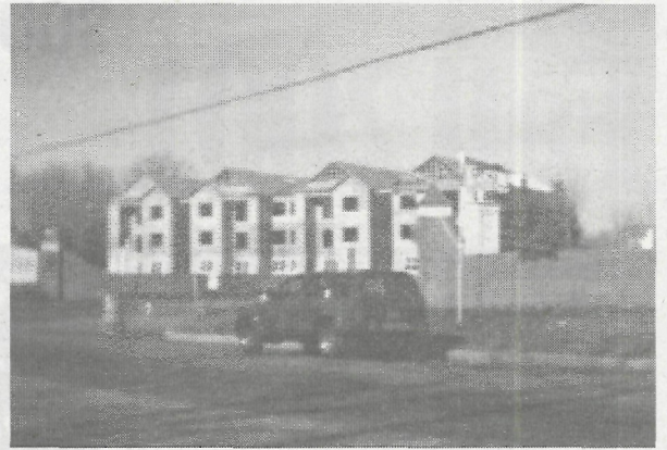
The Senior Housing Complex located on Morris Ave. is beginning to take shape and should be ready for occupancy by spring of 2002.
